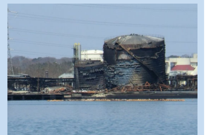
Figure 5: Burned tanks at the Sendai refinery hit by the tsunami (Photo Credit: C. Scawthorn)
